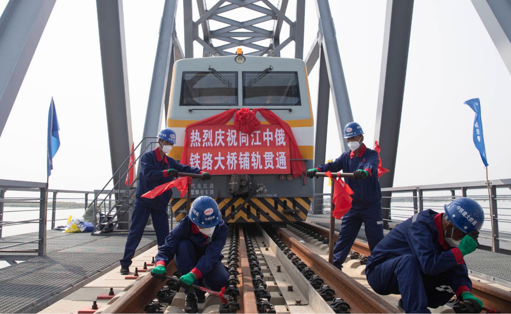
Photo: Constructors work at the construction site of the China-Russia Tongjiang-Nizhneleninskoye cross-border railway bridge, Aug. 17, 2021. The construction finished its tracklaying work on Tuesday. The railway bridge, with a designed annual throughput capacity of 21 million tonnes, connects Nizhneleninskoye in Russia with the border city of Tongjiang in Heilongjiang. Credit: Imago/Alamy
