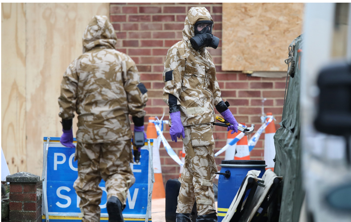
Members of the military wear protective clothing as work continues on the home of former Russian spy Sergei Skripal in Salisbury, Wiltshire. The property is to be dismantled, with the roof completely removed by military teams in the wake of the Novichok attack as decontamination work continues. AP-Images via REUTERS.
